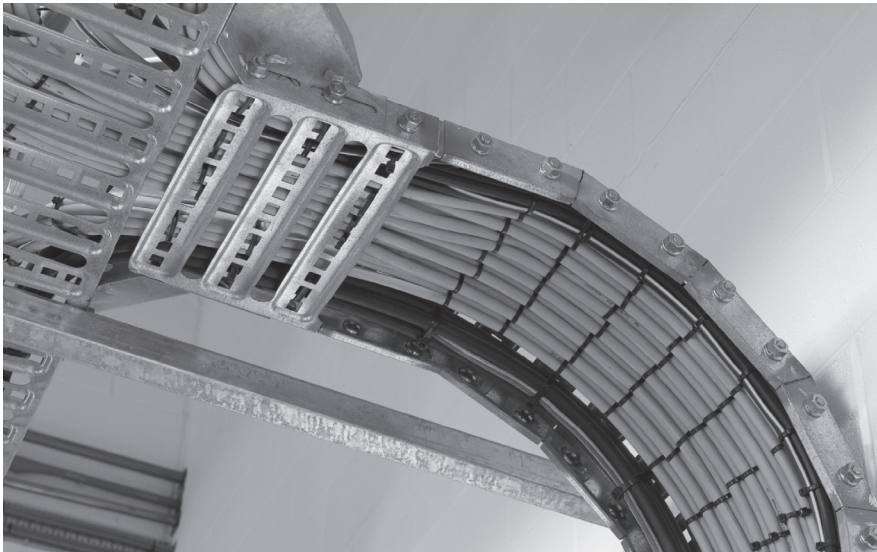
Figure 13.14 Network cable ladder rack
